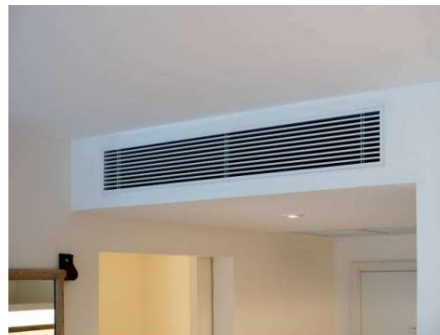
Air conditioning supply grille
